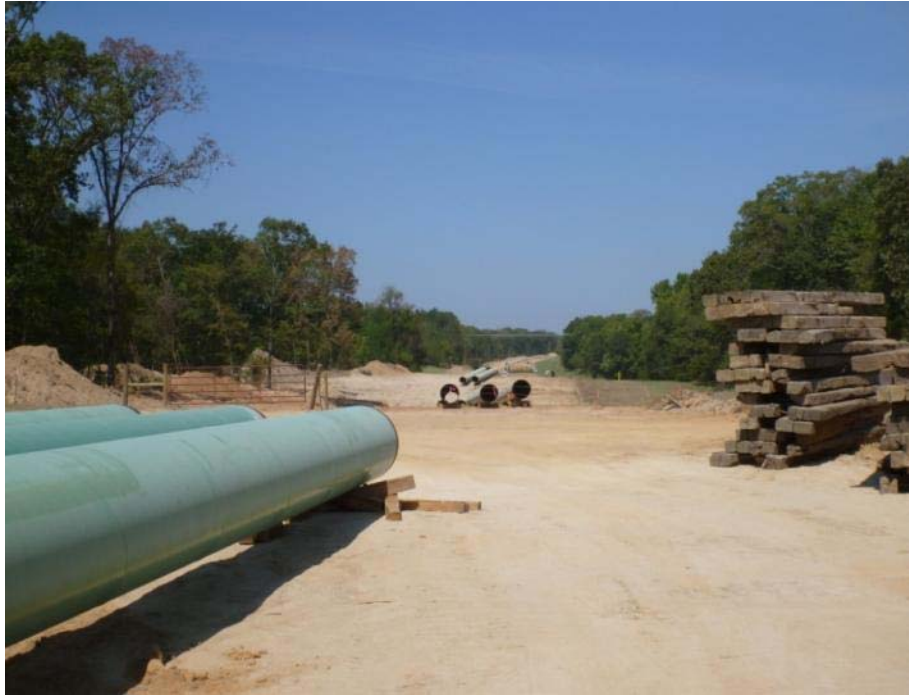
Keystone XL Pipeline Gulf Coast Segment 2 under construction, Northeast Texas September 2012. Photo: HDR Engineering, Inc.
