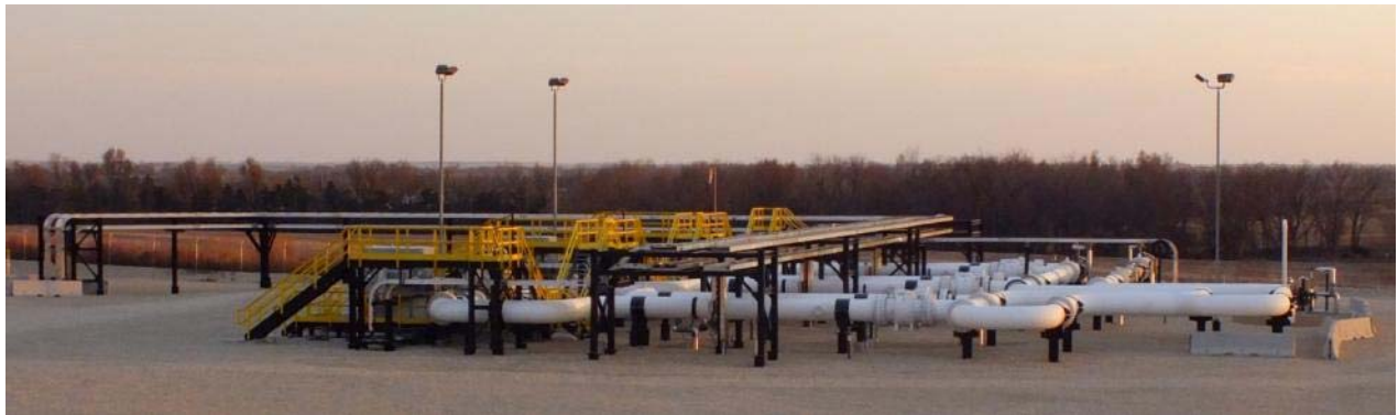
Keystone Oil Pipeline pump station, near Hope, Kansas. November 2012. Photo: NDEQ
